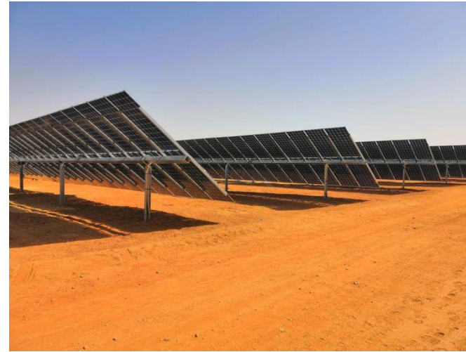
Bifacial PV plant, Egypt
