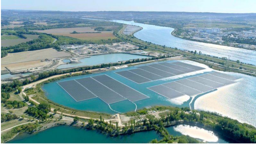
Floating PV plant, France
