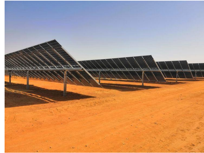
Bifacial PV plant, Egypt
